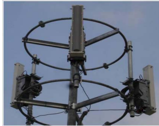
Fig.18:: The 3-sectors BTS antenna installation.
